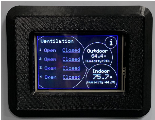
Fig. 5. Controller Main Screen
