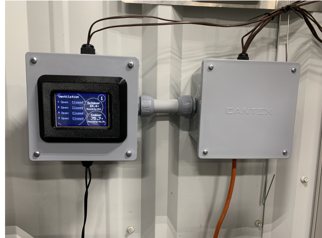
Fig. 10. Controller Final Installation
